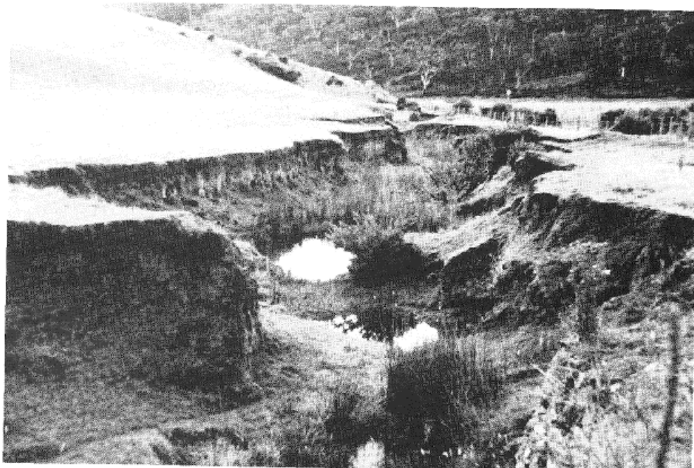
Streambank erosion beside the Cockatoo Gully Road in the Huntingdon Tier (278142) Land System.
