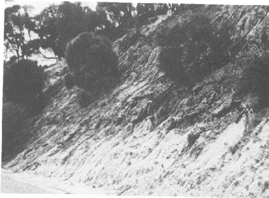
Rilling problems on a road-cutting in the Killora (373143) Land System near Dennes Point.
